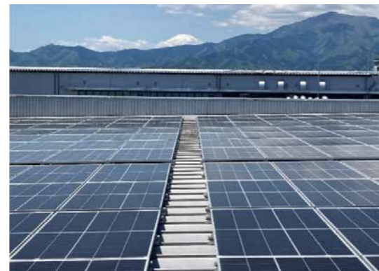
Photovoltaic system (Ebina Plant)
