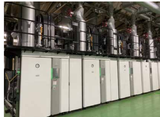
Boiler system (Taiki Plant)
