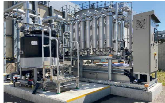
Backwash water recovery equipment (Ebina Plant)
