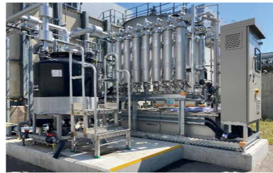
Backwash water recovery equipment (Ebina Plant)
