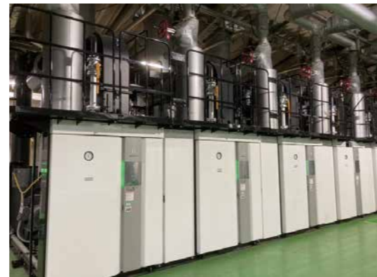
Boiler system (Taiki Plant)
